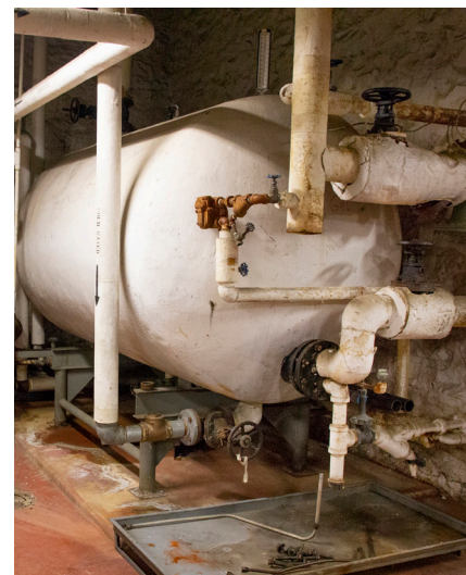
Boiler serving Guild Center
